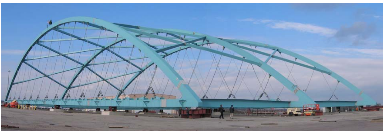
Fig. 31a shows the steel skeleton of the network arch at Providence before it is floated to the site
