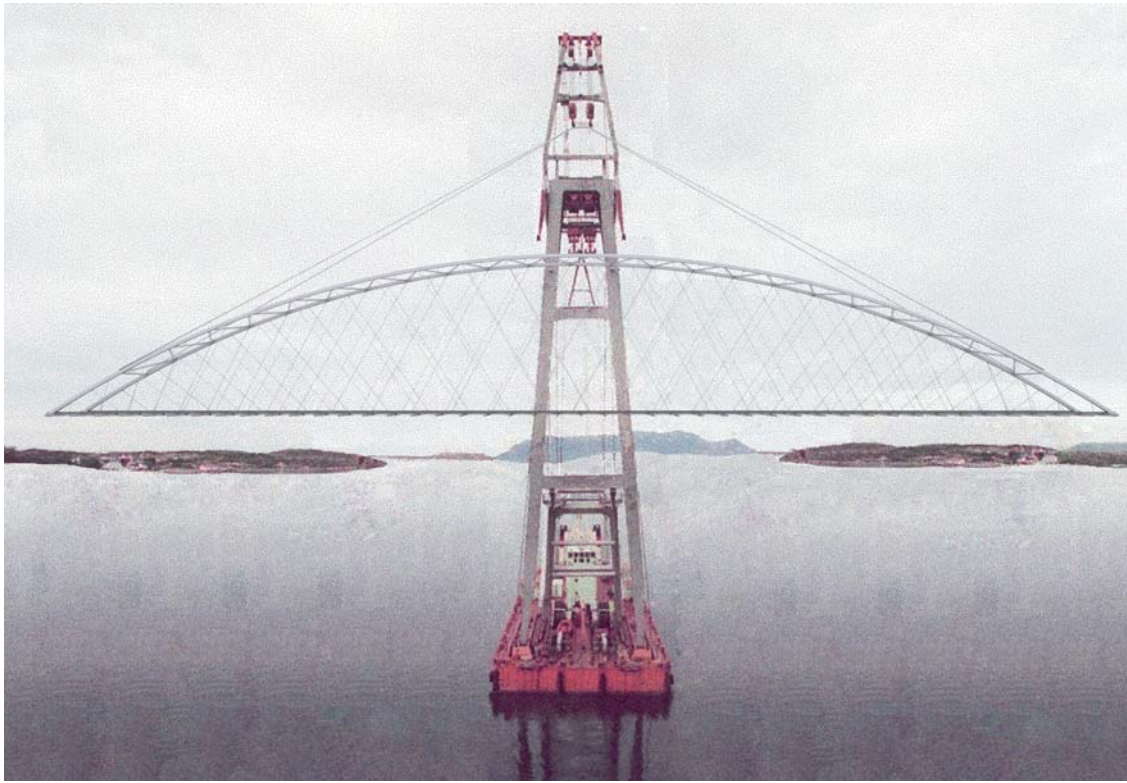
Fig. 39. Lifting the temporary steel skeleton of the Åkviksund Bridge in fig. 97. Span 135 m.
