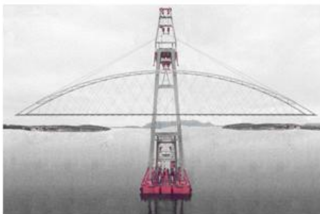
Fig. 33. Lifting the steel skeleton of a network arch with a floating crane.
