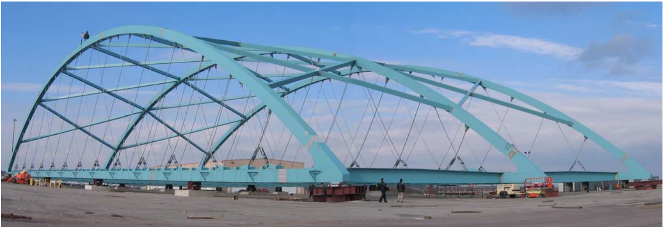
Fig. 50. The steel skeleton of the network arch in Providence ready to be moved.
