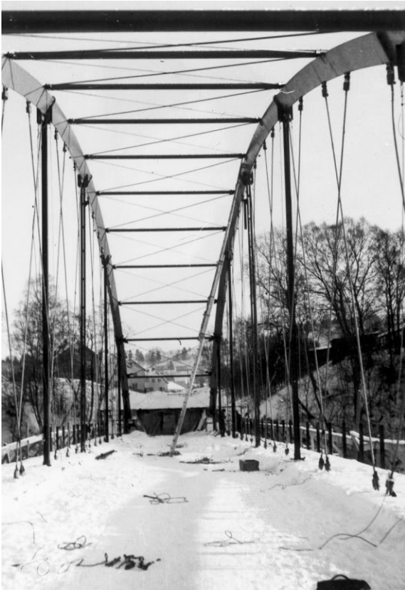
Fig. J9. Erection of arch and hangers at Steinkjer in the winter of 1962-1963
