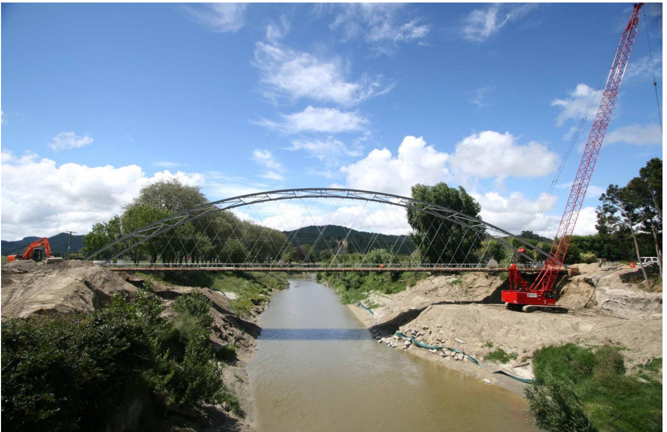
Fig. J20. Steel skeleton of the Mangamahu network arch that was lifted in place by mobile cranes
