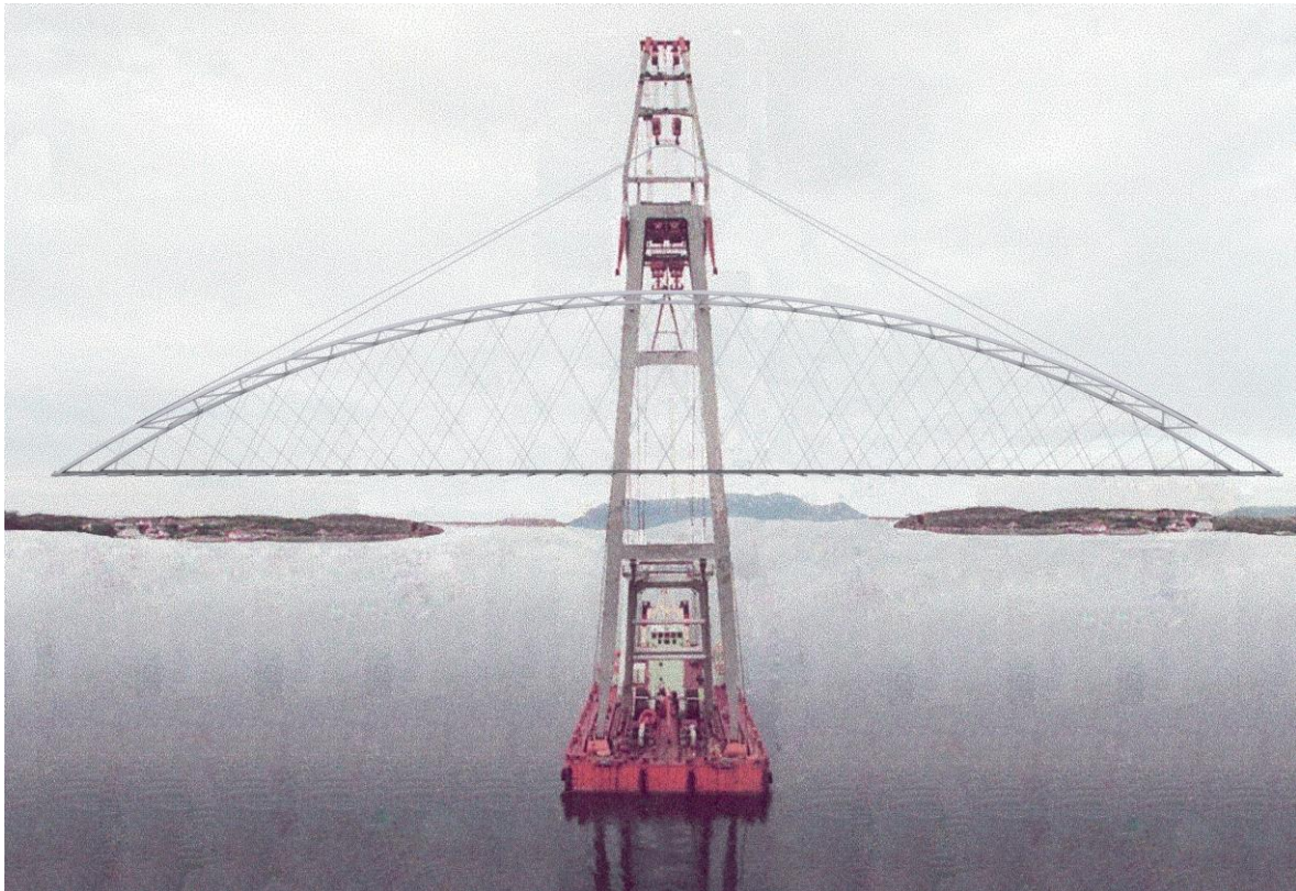
Fig. 39. Lifting the temporary steel skeleton of the Åkvik Sound Bridge in fig. 97, p. 93. Span 135 m.
